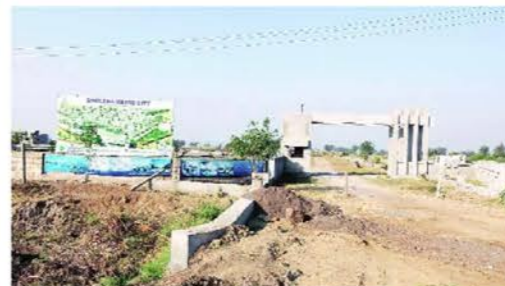
The government has put in money in Dholera and "will continue to put in money", he said and added 95 per cent land acquisition has been completed for an Expressway between Ahmedabad-Dholera. (Source: File)
