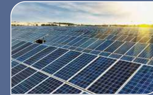
5000 MW POWER PLANT AND SOLAR PARK
